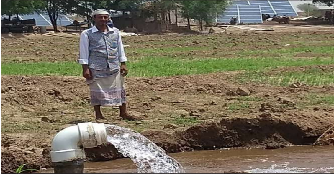
Irrigation solar pump project, AL Solemanah village, AL Mrawa District, Hodeidah (Photo Credit: AFCAR)
