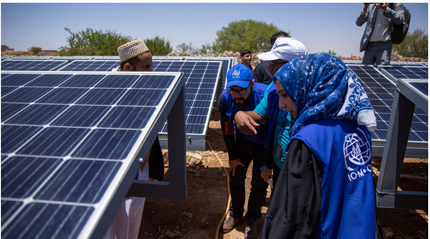
IOM GIVES A FINAL REVIEW BEFORE HANDING OVER A SOLAR WATER PUMPING SYSTEM TO A CONFLICT-AFFECT COMMUNITY IN AMRAN GOVERNORATE. ©IOM 2019/HEADON
