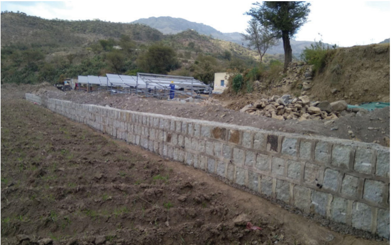
Retaining walls were built at the well to protect against water flooding. Zameh, Ibb. Photo: UNOPS 2023.
