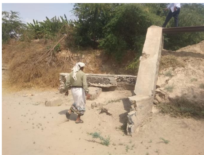
Photo 3.1 Damaged control gate and gates frames Wadi Bana, Abyan | Photo Credit: UNDP, March 2022
