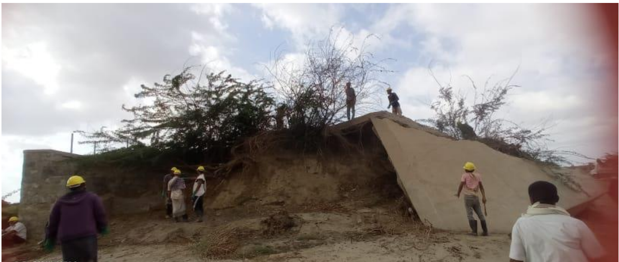
Photo 2.2 CfW on large, damaged irrigation structures, Abyan | Photo Credit: UNDP, March 2022
